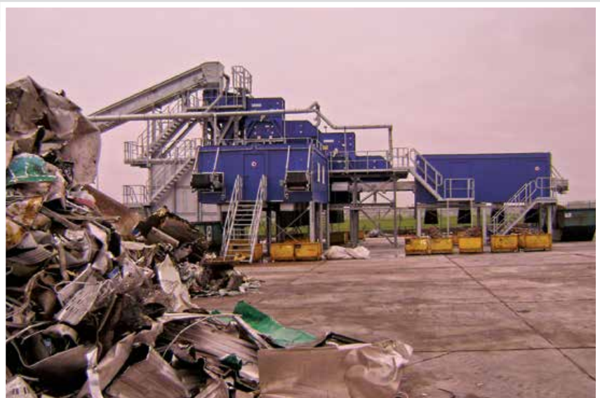
Rumania electronic waste processing plant
