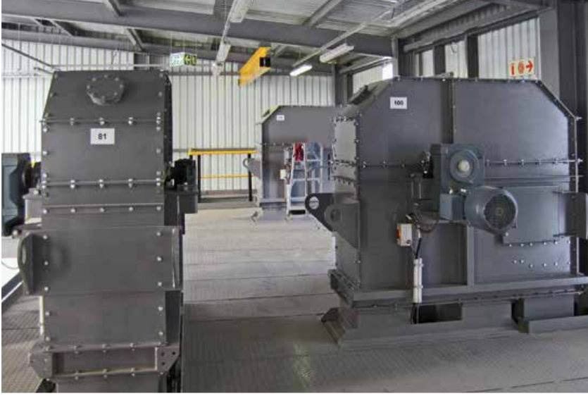
South Africa glass processing system – bucket elevators
