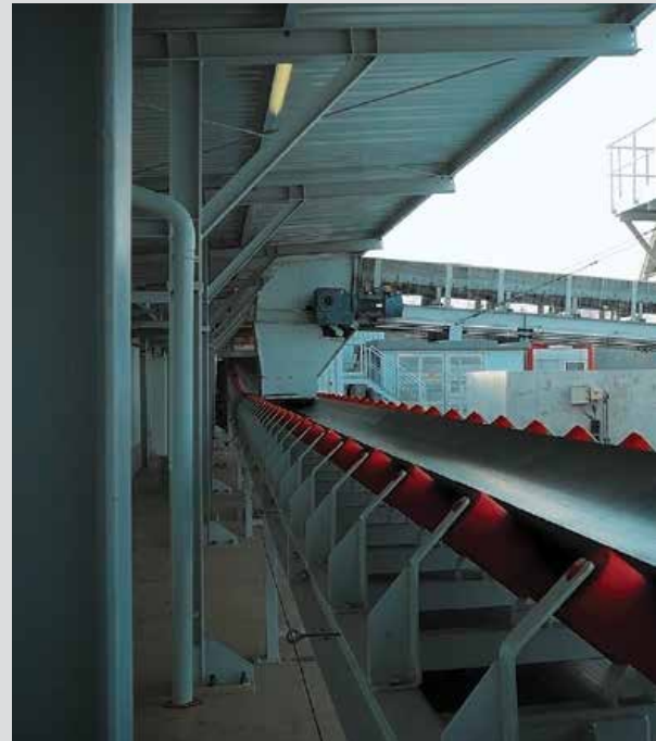
Austria Dürnrohr Power Plant
