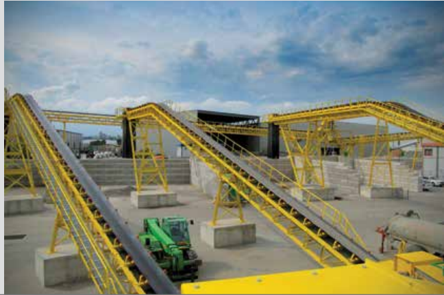
Germany feeding hopper with belt feeder
